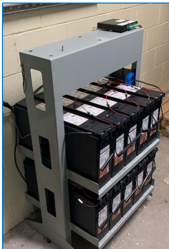
Standard Installation on battery rack
