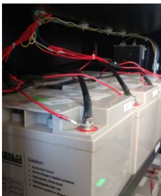
Inside Battery Cabinet
