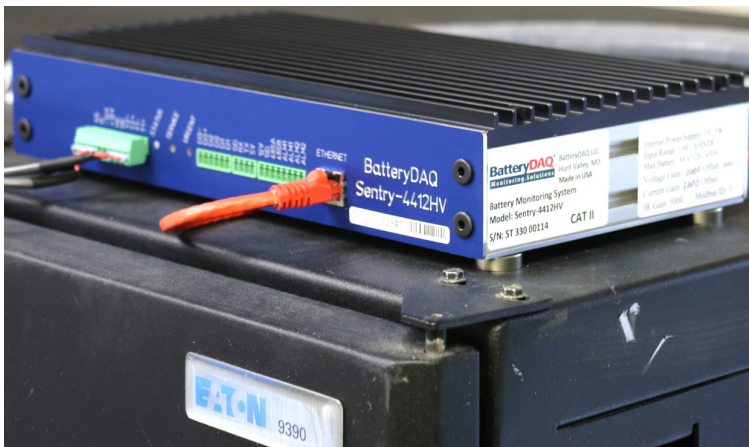
On Top of Battery Cabinet
