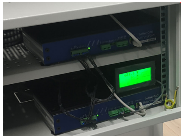
Inside Additional Enclosure
