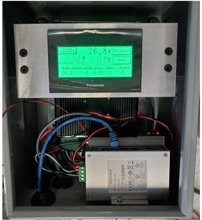
HMI inside steel enclosure. (Moxa Ethernet and Modbus to collect data from GenPro and Genset controller)
