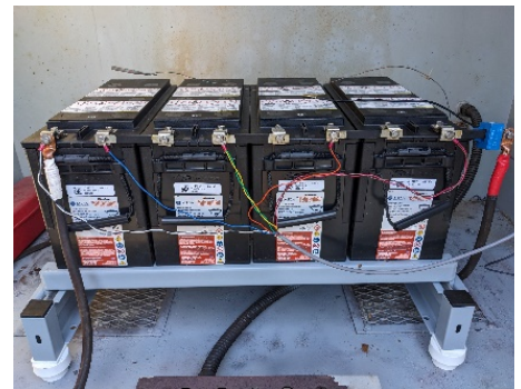
Substation Support System
