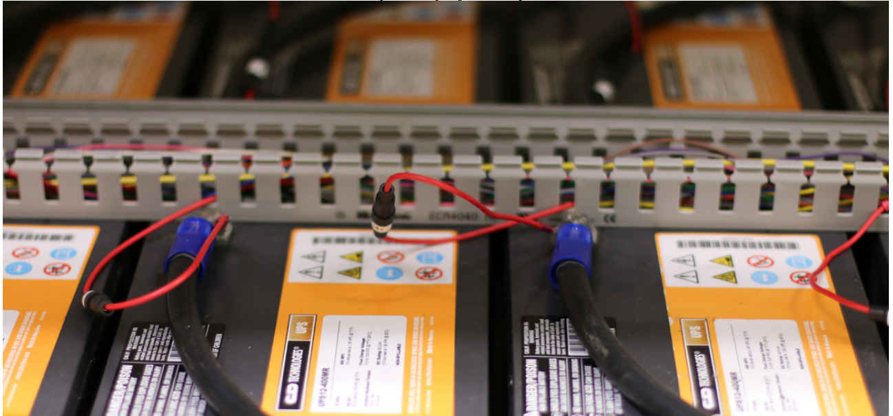
Cable tray on top of battery blocks
